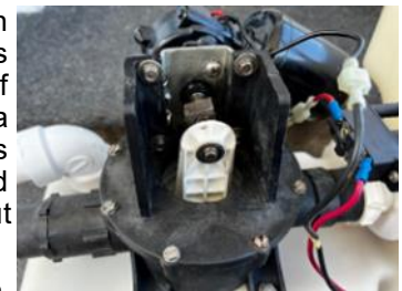
Vacuum generator assembly
